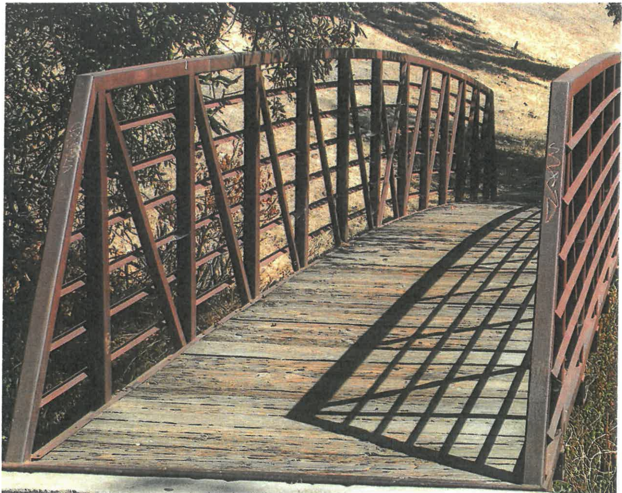
Before – decay wood
